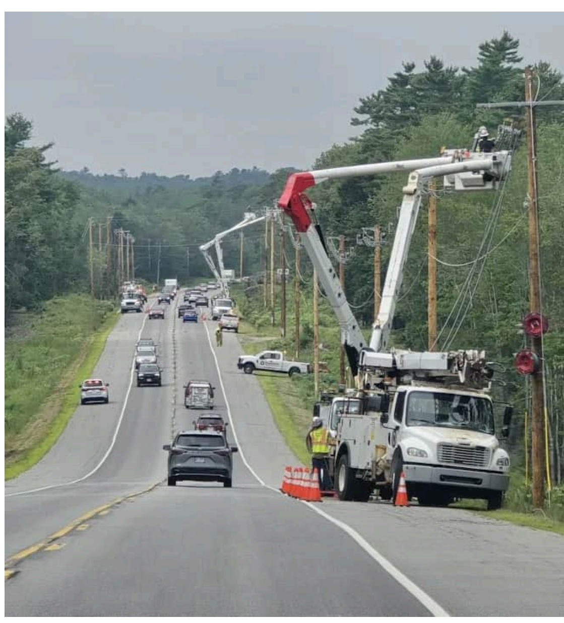
Safety is always our priority. Here crews work along busy Route 1 in Woolwich.
