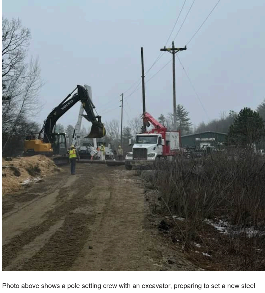
Photo above shows a pole setting crew with an excavator, preparing to set a new steel pole in Sanford in April 2025.
