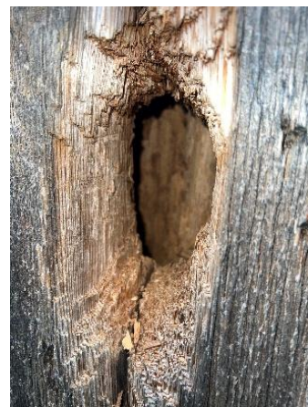
Figure 35. Cavity in a Wooden Pole Left by a Woodpecker in the CMP Service Area
