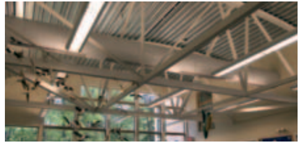
Sleek fluorescent fixtures provide direct and indirect lighting using energy efficient T-8 lamps. This provides bright, uniform lighting, while minimizing glare.
