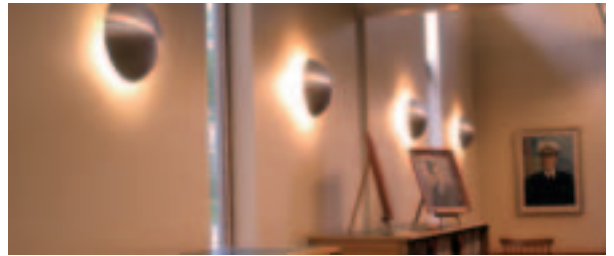
Decorative wall sconces use compact fluorescent lamps to provide wall-washing illumination with an interesting eye-catching fixture.
