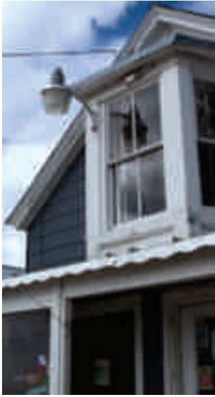
Mercury vapor light at front entrance is old and inefficient
