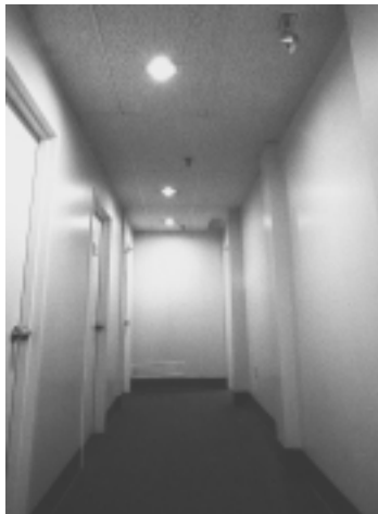
Compact fluorescent lamps in recessed fixtures provide economical and pleasing
